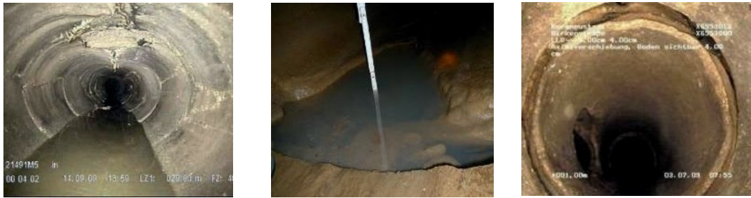
Figure 5: Application examples for the tight-in-pipe method. Left: Deformation (AZ IIIa), Middle: Breakout at the pipe invert (AZ III), Right: Missing pipe piece (AZ IIIa).
